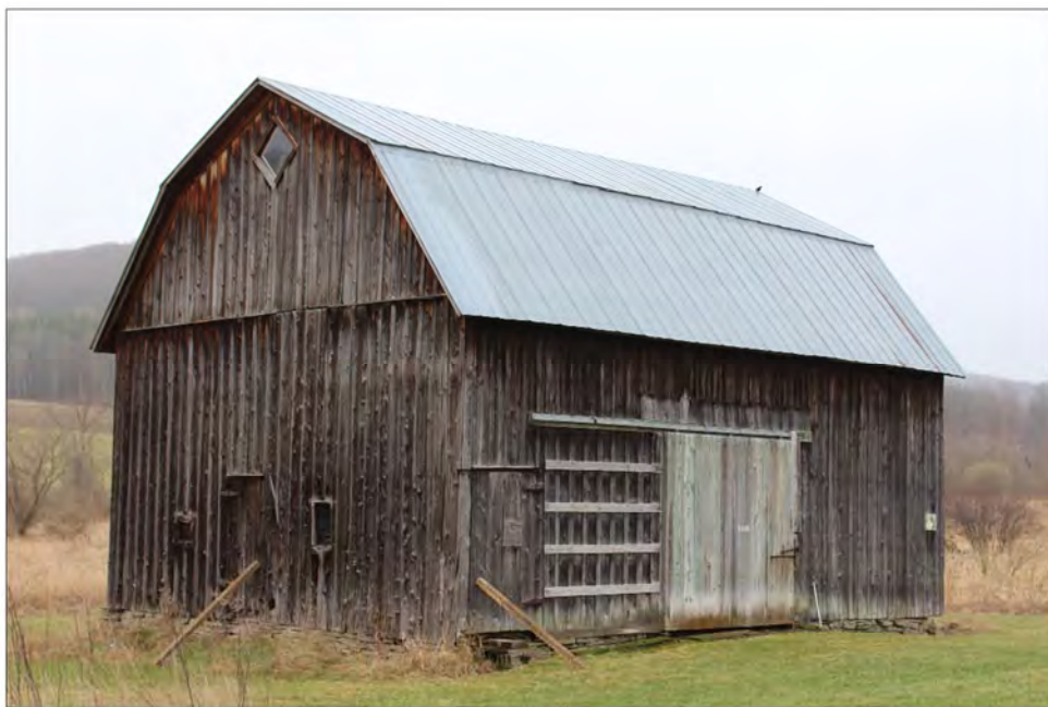
Photo 7.18: Typical late nineteenth- or early twentieth-century side gambrel barn on ground-level foundation (TRC# 1694) (Philip A. Hayden, April 6, 2017, Image# 721).
